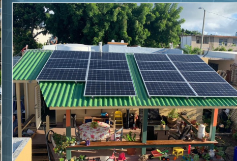
4.5 kw + Battery Backup System, Gurabo
